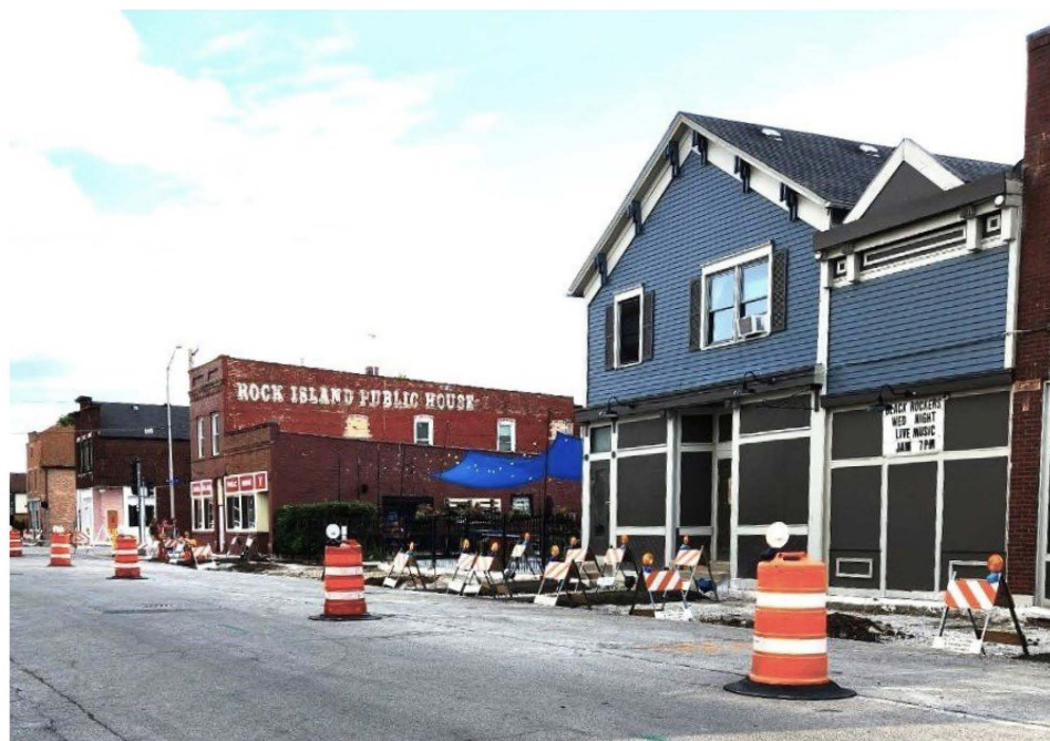
Construction is ongoing along Old Western Avenue in Blue Island, where a project aims to make the area more pedestrian friendly. CAROL FLYNN/DAILY SOUTHTOWN PHOTOS
